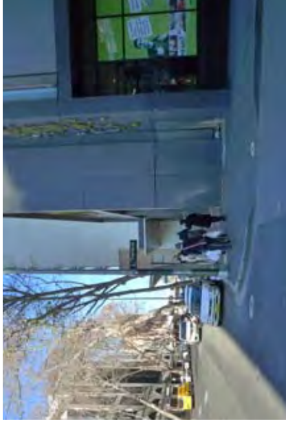
Narrow footpath due to large kerb indent at 'Urbanest' (southwestern corner of Thomas Street intersection)
