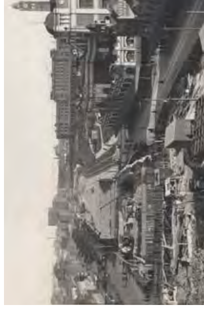
Belmore Park 1923, during construction of the City Circle railway lines (source: Tyrell Collection, Powerhouse Museum)
