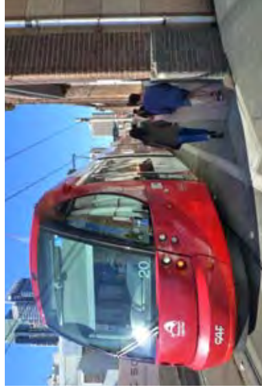
Insufficient footpath width between UTS Building 5 and light rail lines at the western (Darling Drive) end of Hay Street
